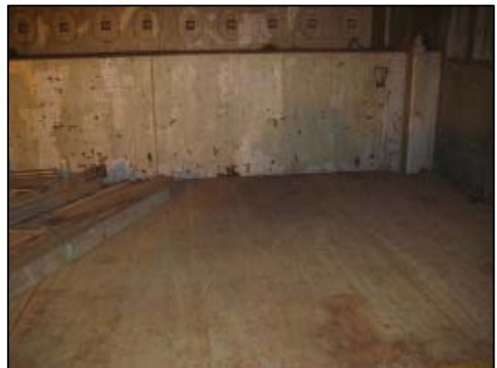
Skid marks from the moving bins
